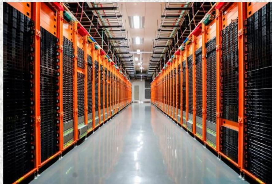
Figure 9: An Alibaba data center [5].
