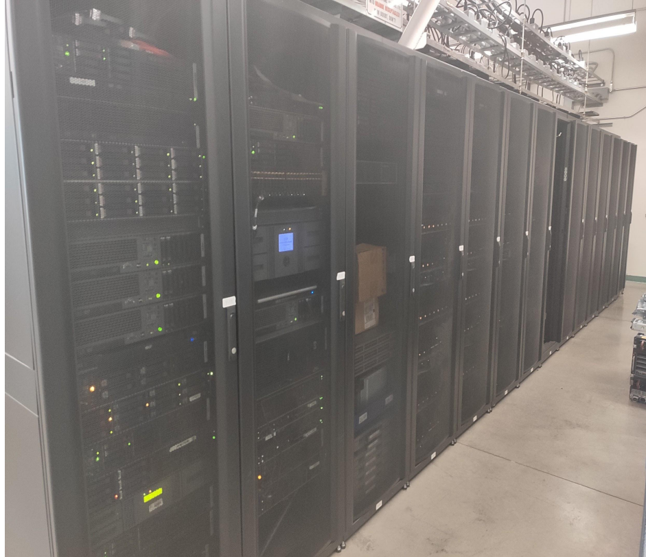
CSUN MDF Server Racks
